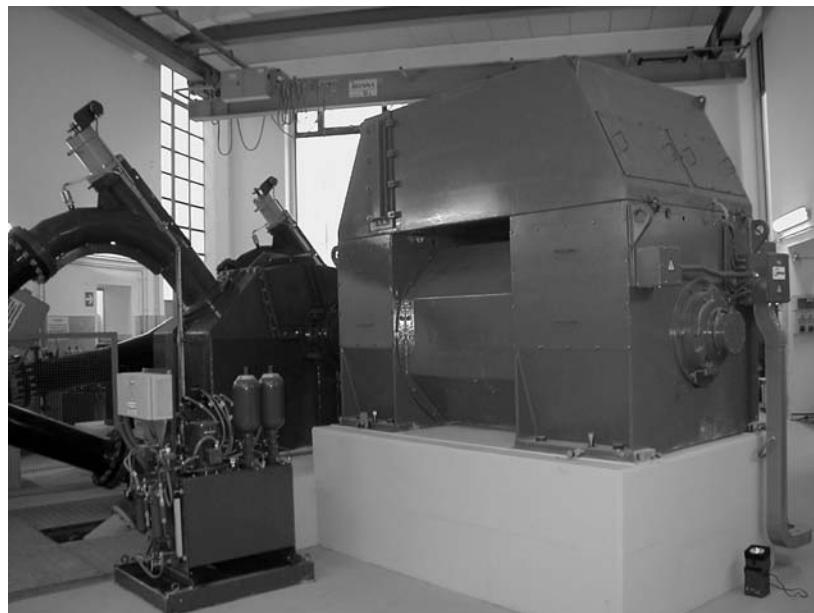
Fig. 2: the machine hall after upgrading
