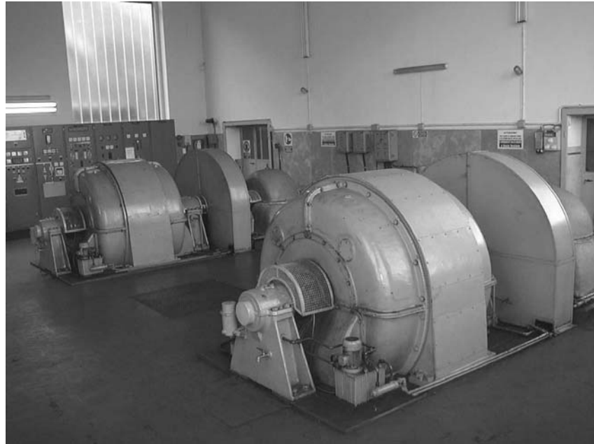
Fig. 1: the machine hall before upgrading
